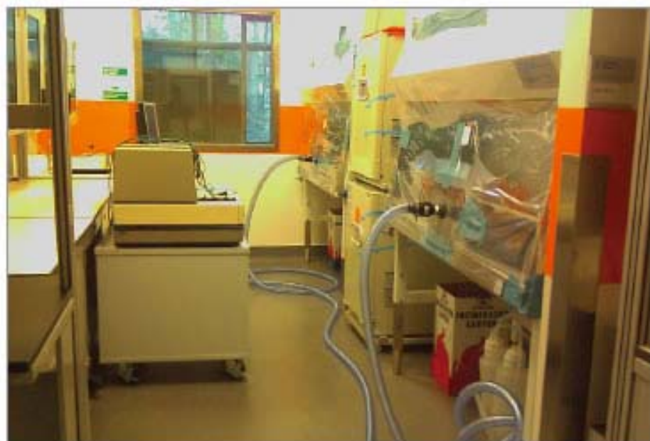
Figure 1: Decontamination Equipment Attached to BSCs
