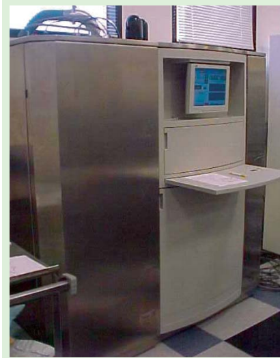
Photo 1: Isodox chlorine dioxide gas generator
